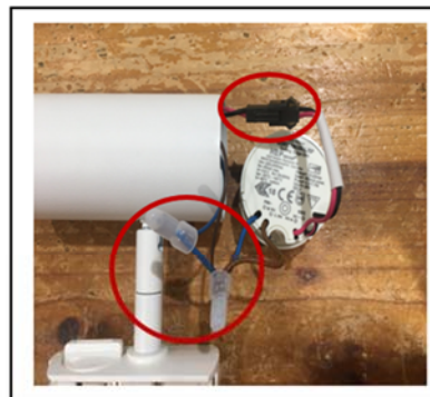
Figure2 Loose the connection
